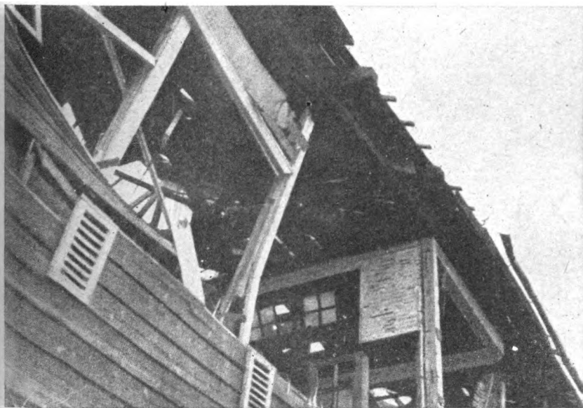
Figure 5.66a. Upper photo: Wood-frame building, 8,000 feet from ground zero, showing rupture of columns at points where windows or other horizontals were mortised in. Lower photo: Detail of above, showing typical column failure. (Note mortise and tenon joints at wall plate.)
